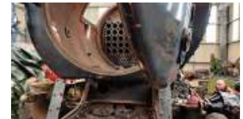
The front end. Still to be fitted are the double chimney, the Kylchap blastpipe, the superheater, the ash baffles, and the central Caprotti box.
