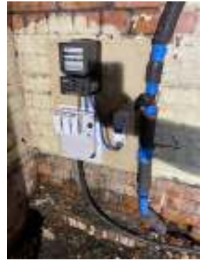
The new 3 Phase supply installed at Henley-in-Arden
