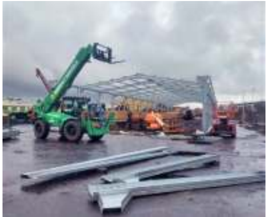
View from the Warwick Road end showing the platform demolition and steelwork erection.
