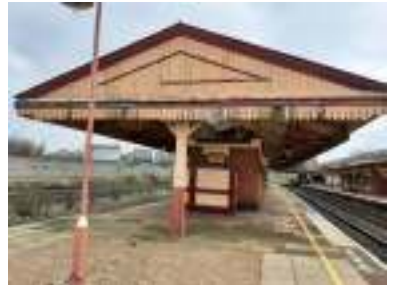
The dagger boards at Tyseley, in urgent need of renewal
