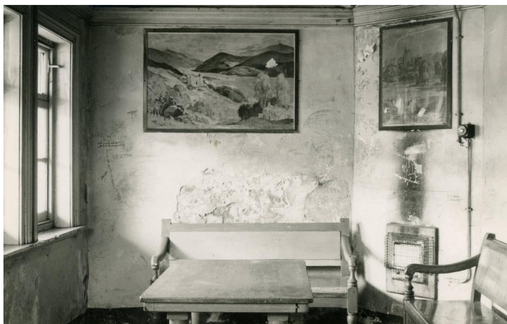
Keeping the Shakespeare line in mind, this photograph from the archive shows Hall Green station down waiting room with pre-war travel posters on the walls, peeling plaster and a 'modern' electric fire with a trail of soot up the wall, plus GWR furniture. Feb 1970 Image C.C. Green
