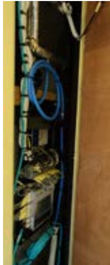
The 'brains' of the toilet. This is the bit you do not usually see. In the panel behind the toilet this small computer controls the water supply, compressor, and warning lights. If it senses anything out of order, it shuts the system down. The wire at the top right of the picture goes to the 'out of order' light
