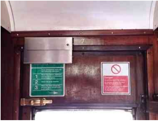
24v dc volt door locking bolt mounted on Mk1 coach door.
