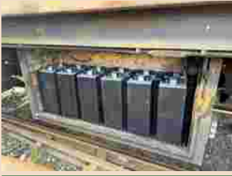
One set of the new batteries in place in the Kitchen Car. Photo: Alan Brookes
